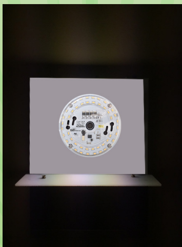
Focus Retrofit Install 1x 13w LED 14w Total per Fixture
