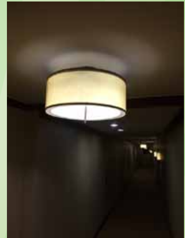
Focus Retrofit Install Is Identical In Color & Light Output With 25w Energy Savings Per Fixture
