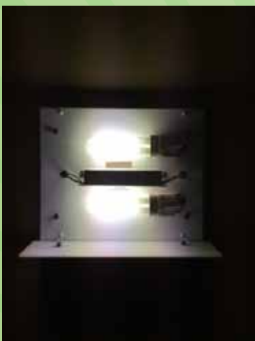
Original Install 2x 13w CFL 26w Total Per Fixture
